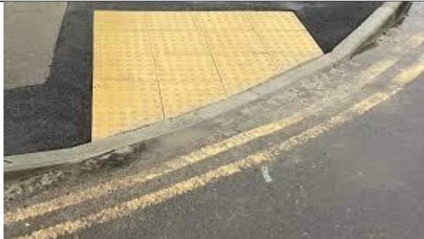
Absence of dropped kerb at crossing point
