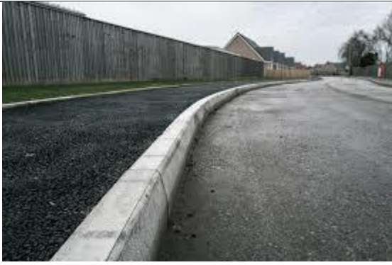
Narrow footway due to street clutter (under 1.5m)
